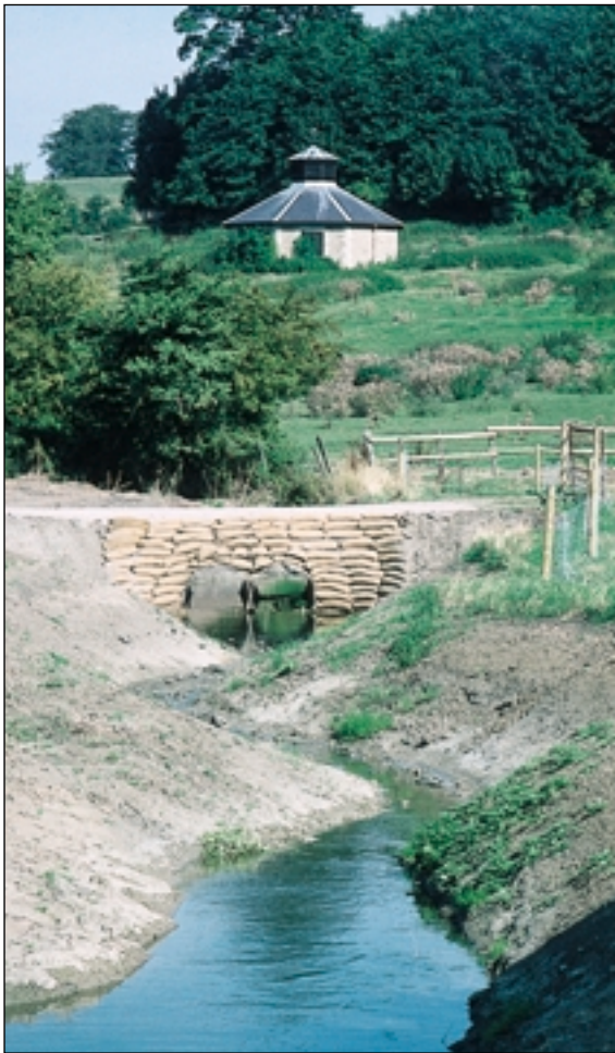
Flood drain crossing seen from bank of R. Cole. (bagwork wing walls incomplete)
