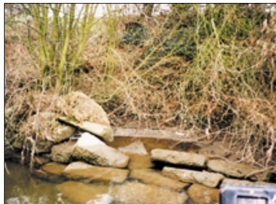
Failed section of bagwork at Clifton Lock Cut
