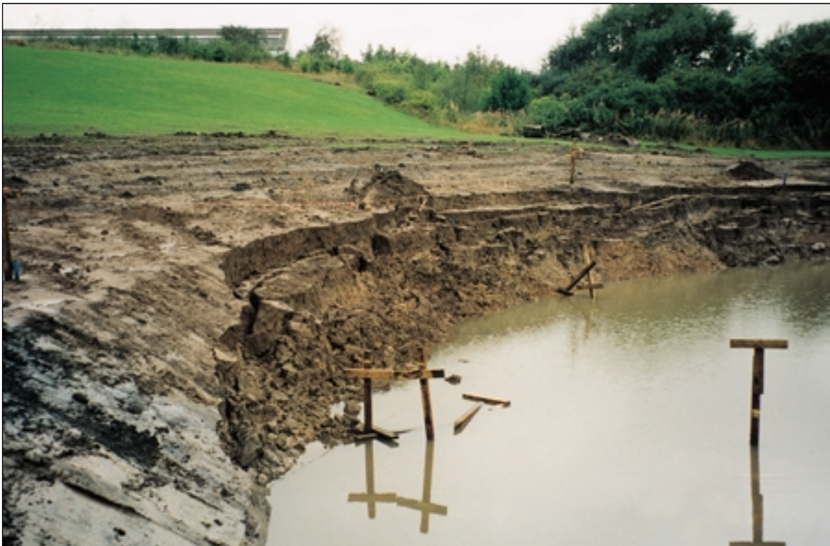
Slipped slope during work – September 1995
