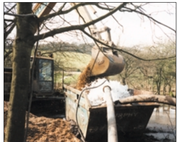
Pumping apparatus in operation
