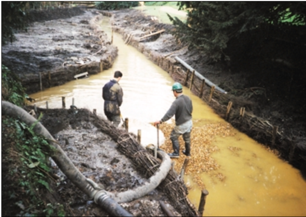
View of the wide dredged section, gravel being placed within the low-flow channel
