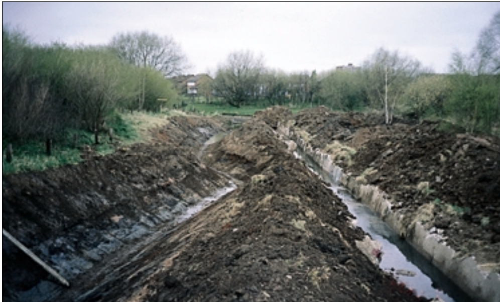
The 'new' Brook being excavated adjacent to the old channel. Spoil stockpiled
